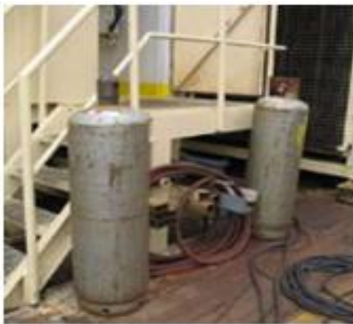
Improper storage of cylinders and set up of the cables
