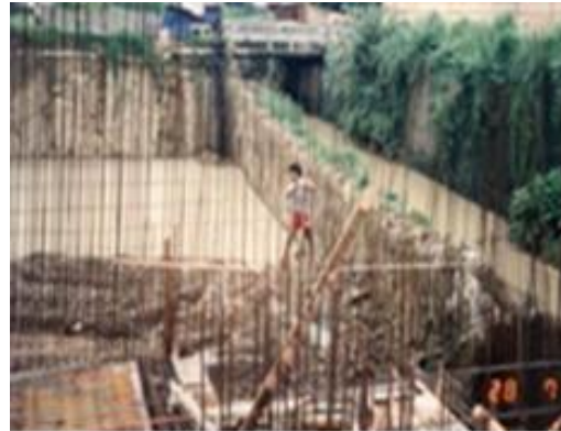
Workers without any safety harness other safety gadgets for working
