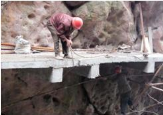
Workers without safety gloves and and safety harness working
